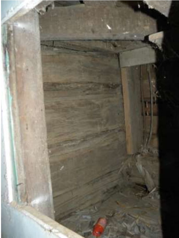
Exposed logs under stairwell.
