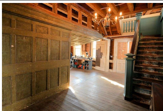
Hinged panel wall after restoration work. One panel is down and the other up in this photo.
