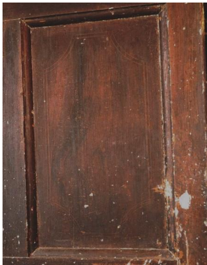
Panel detail showing faux mahogany finish on yellow pine lumber.
