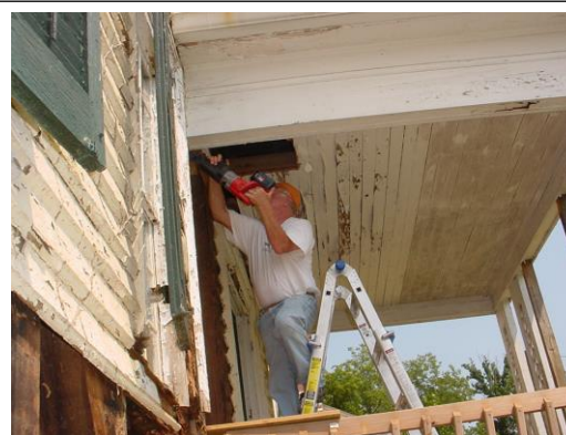
Ray Carney works to stabilize a deteriorated beam in order to lock the double doors.
