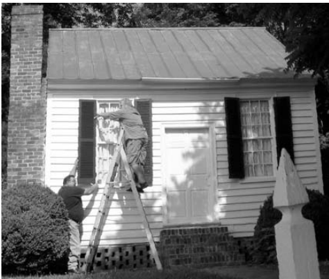
VOLUNTEERS DOUG CORDARO AND CARL BIGNESS INSTALL SHUTTERS AT THE HISTORIC MANLY LAW OFFICE
